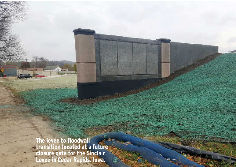
Construction of the Sinclair Levee, a former Brownfield site in Cedar Rapids, Iowa.
