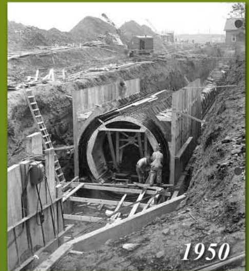
Philadelphia began replacing wooden pipes (top, wooden pipes uncovered ca. 1900) with cast iron ones (middle, 1904) in the 19th century. Besides being more durable, the cast-iron pipes made it easier to maintain water pressure throughout the system. Today's distribution system contains pipes made of cast-iron, ductile iron, steel, and concrete. The large concrete Queen Lane pipe shown above (bottom, 1950) carries water from one reservoir to another.
